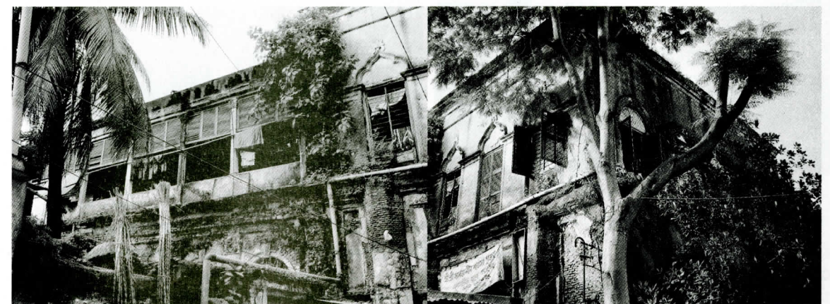
Figure 21: View of the police station and residence from the Shirish Babu lane.
