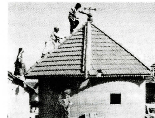
Figure 17: Circular house under construction in 2001 Kutch earthquake rehabilitation exercise. Source: Kotak, 2007, p71.
