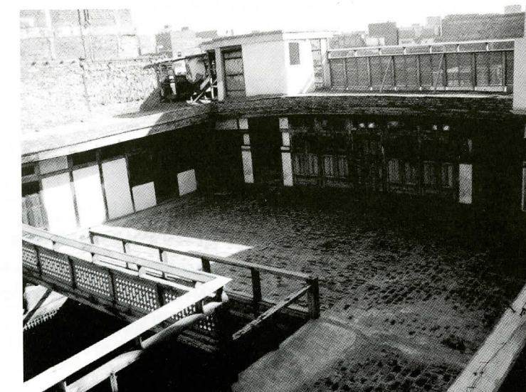
Figure 09: Kitchen and other service areas on top floor, Gul Ahmad Sethi Haveli
