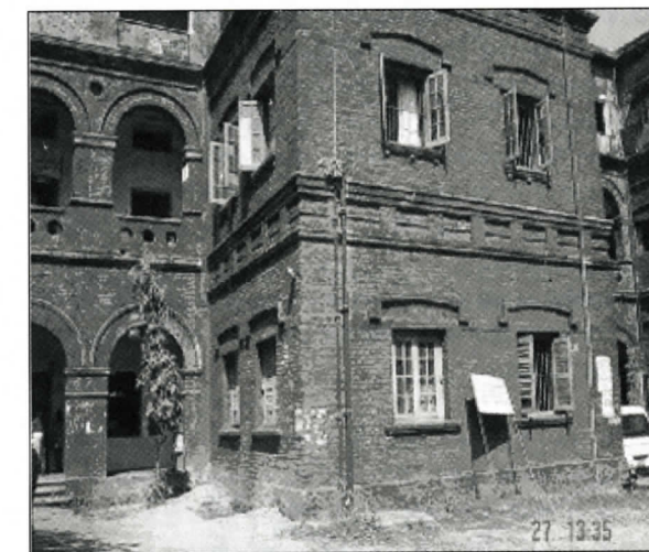
Figure 5b : Treatment of openings in the walls and elevation of Chittagong Court Building.
